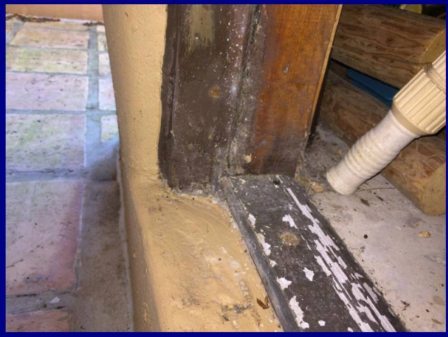
Wood decay lower left door jam, at right exterior closet.
