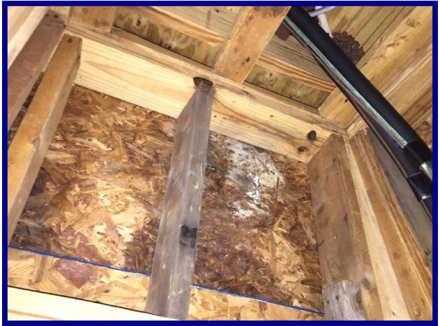
Wood decay at wall sheathing | left exterior closet.
