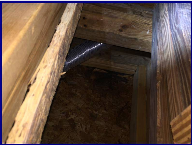
Wood decay at wall sheathing up high in closet right exterior.
