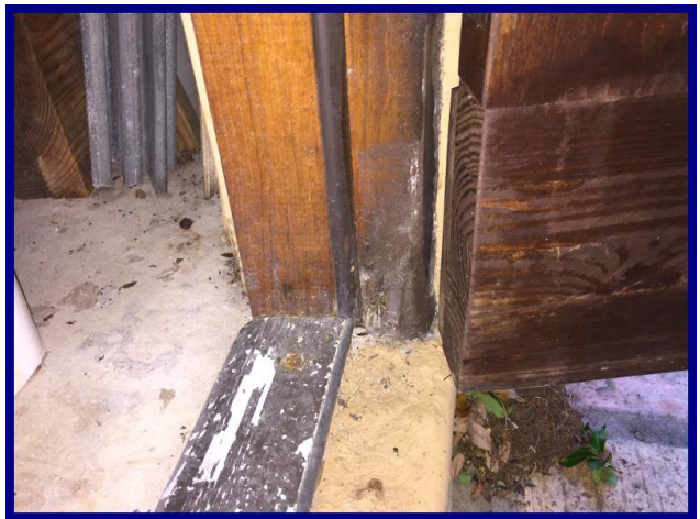
Wood decay at lower right door jam, exterior right closet.
